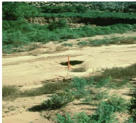
Figure 6. Sinkhole in road in Montezuma Creek, southeastern Utah, caused by collapse of a soil pipe.
