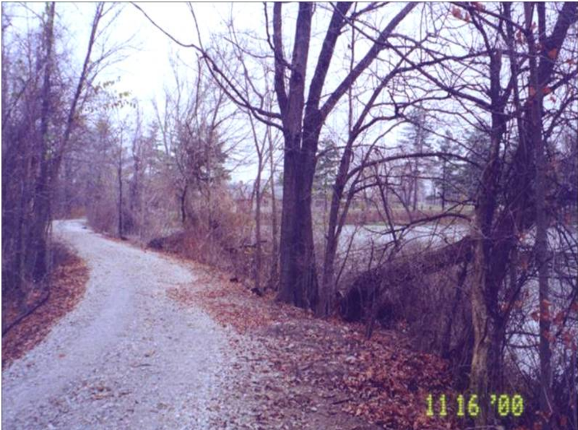
Figure 12. Poorly Maintained Dam.
