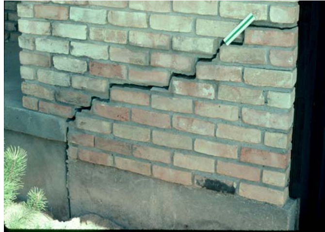
Figure 3. Damage to a house in Cedar City caused by collapsible soil.
