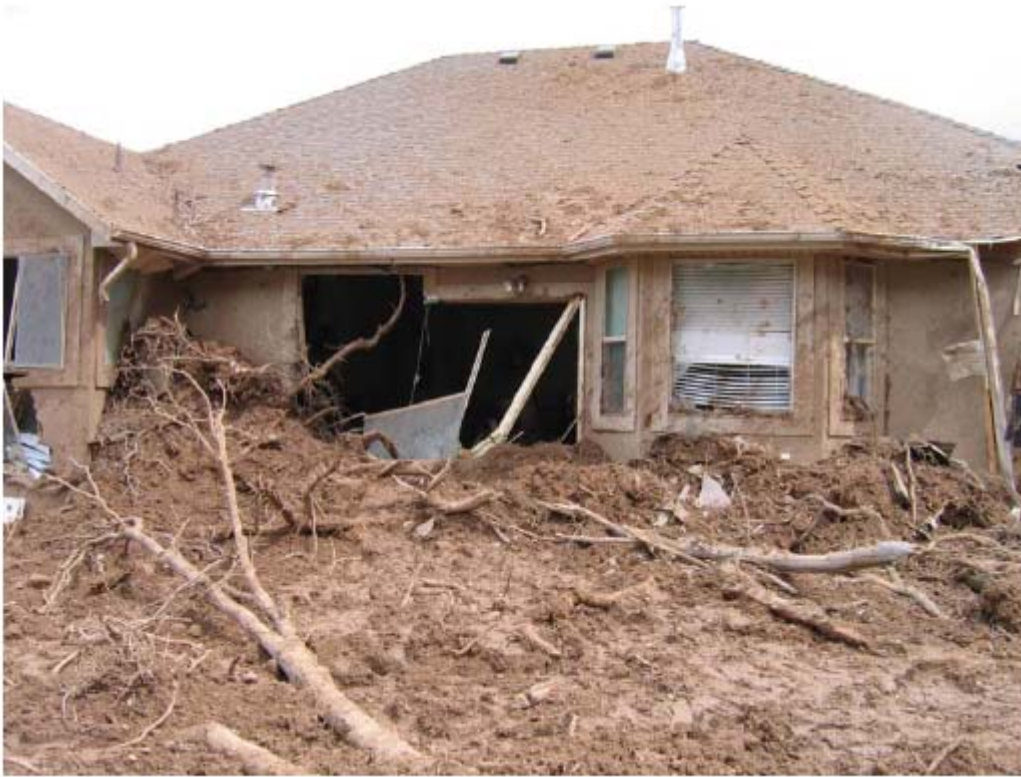
Figure 4. A rapidly moving landslide in 2006 impacted this house in South Weber, damaging the house and injuring a child inside.
