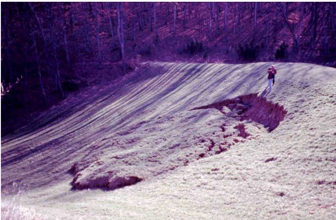
Figure 13. Slope Stability Failure.
