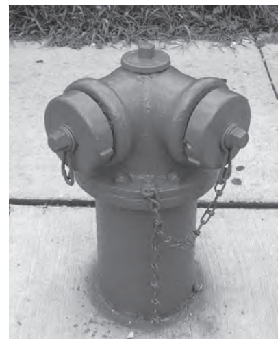
public fire hydrant
